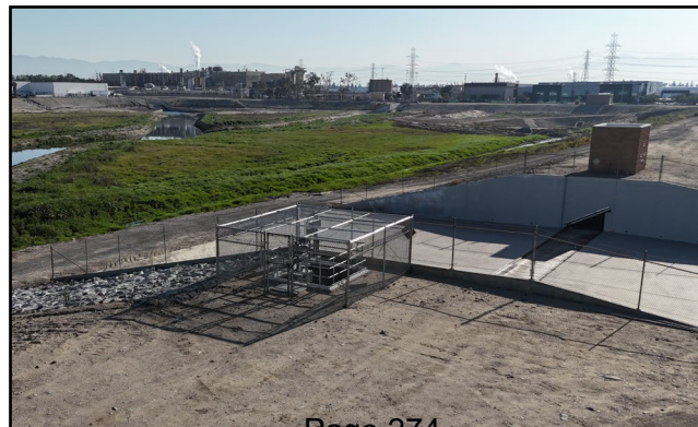
Outlet Control Gate/Rubber Dam System
